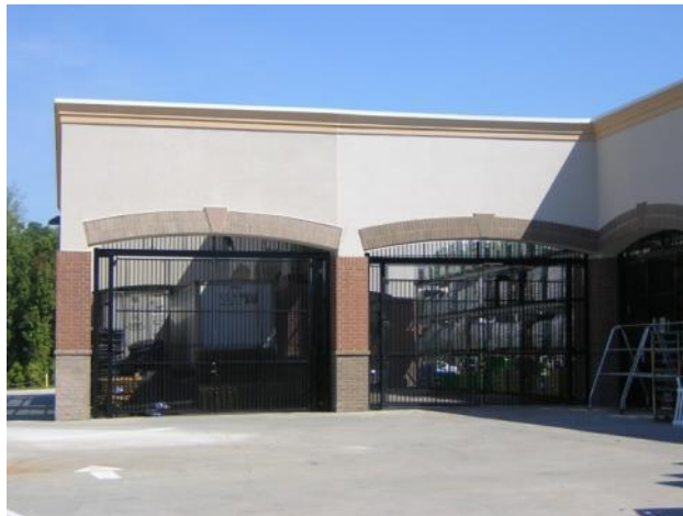
Figure 10.08-B: Use of a wall and fencing for screening that is architecturally compatible with the principal building.
